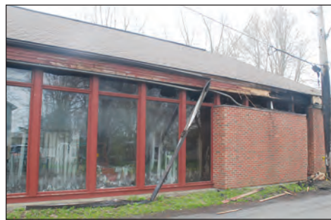
This photo shows the damage to the side of the food bank building, including the scorched hydro pole alongside the back section. Morin Photo
